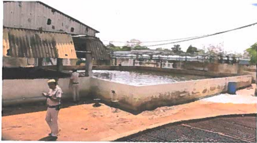
Wazirpur Industrial Area CETP Plant
