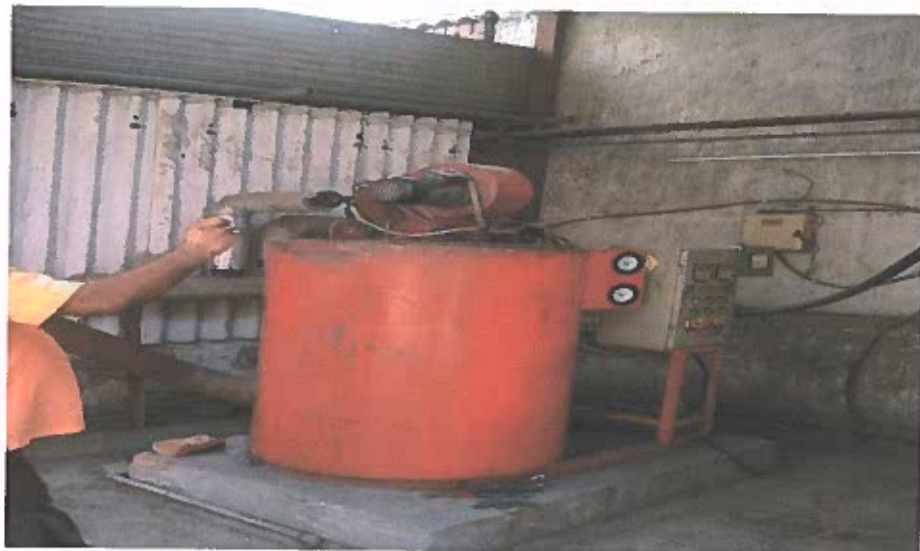
M/s Silkon Thread Pvt. Ltd. (Boiler)
