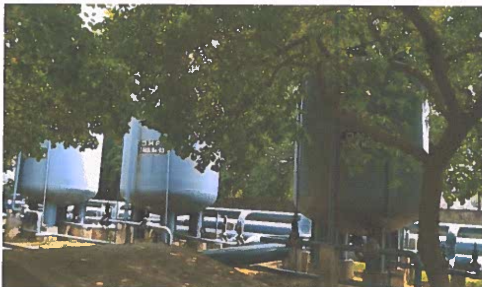
Badli Industrial Area CETP
