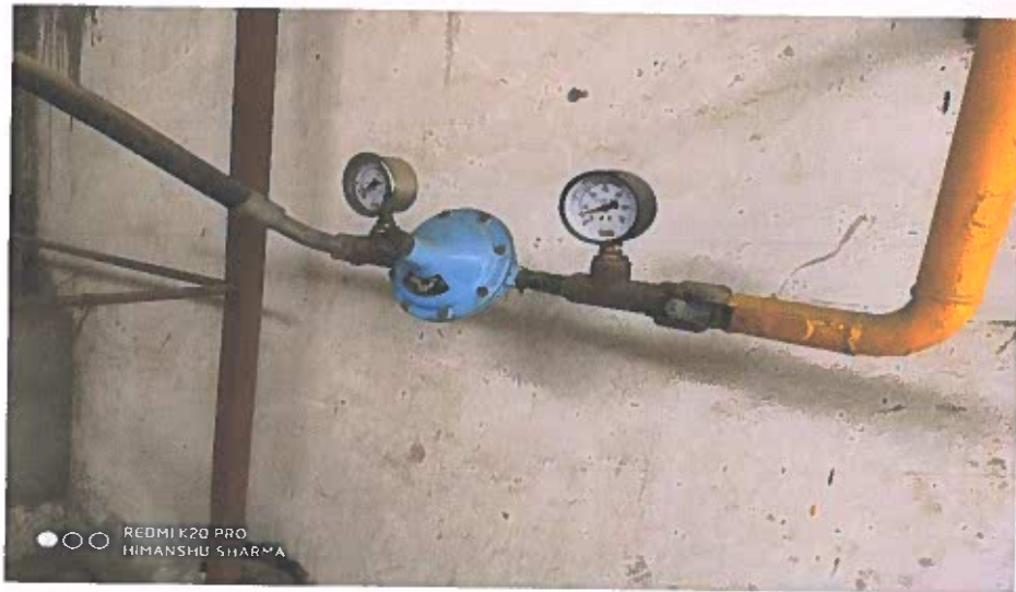
M/s Silkon Thread Pvt. Ltd. (PNG Connection for Boiler)
