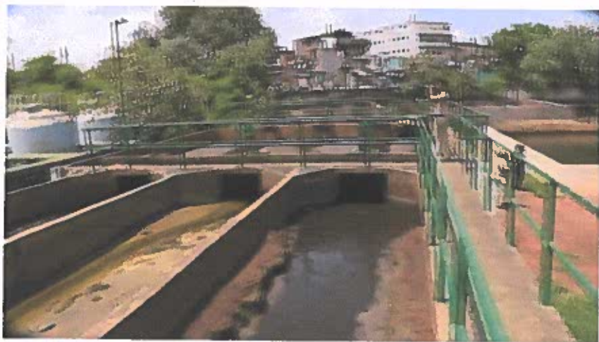
Wazirpur Industrial Area CETP Plant
